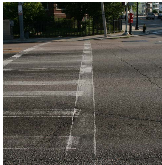
Faded crosswalk at intersection of Morton and Norfolk streets
