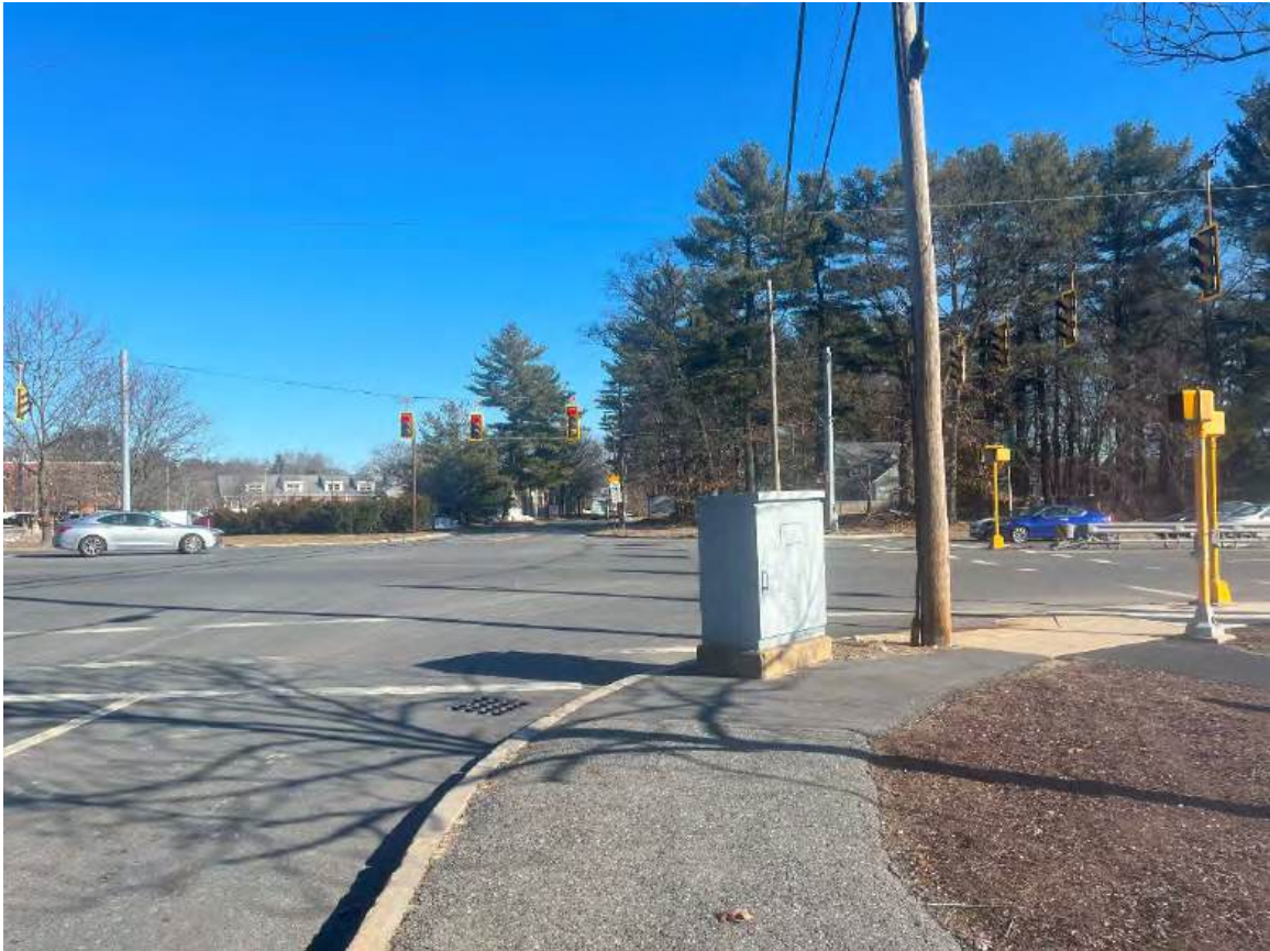
Figure 3 Signal Controller Cabinet on ORNAC
