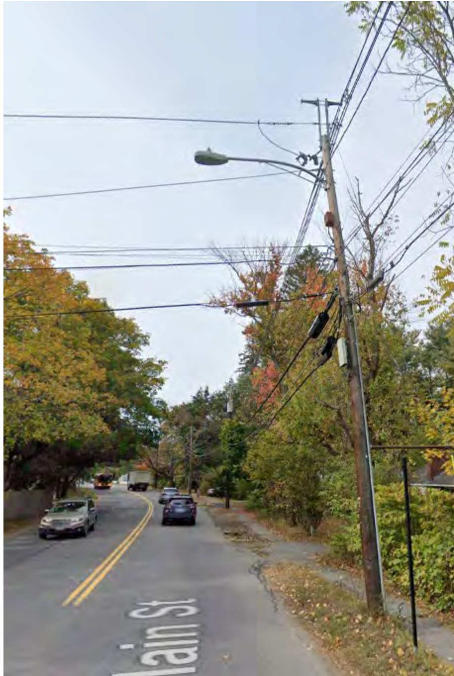
Figure 4 Streetlight on Route 62 Near Orchard Road
