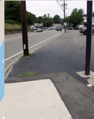
New curb ramps but no sidewalk separation
