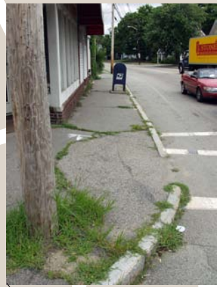
Sidewalk and curb in disrepair
