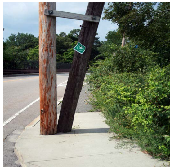
Grove Street NB: overgrown vegetation
