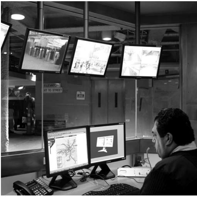
HUB MONITORING STATION
